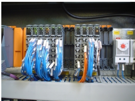
Figure 30: SINCONV connection SINCONV 的连接
