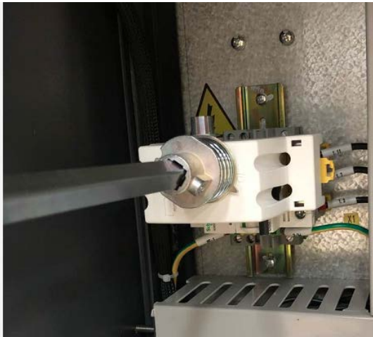
Figure69: Checking operation of ventilation 检查通风操作
