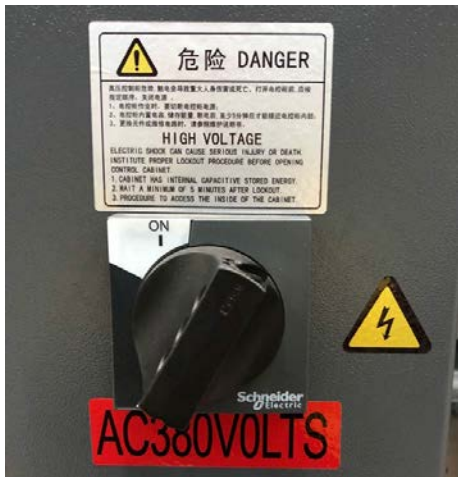
Figure63:Electrical Cabinet ON/OFF switch 电柜 ON/OFF 开关
