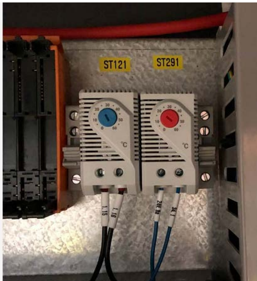
Figure 26: Checking operation of ventilation 检查通风操作
