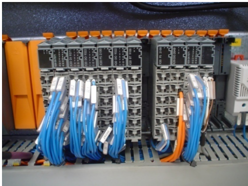
Figure 34: SINCONV connection SINCONV 的连接
