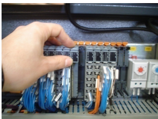
Figure31: SINCONV connection SINCONV 的连接
