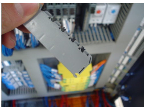
Figure 32: SINCONV connection SINCONV 的连接
