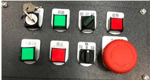
Figure 74:Control Panel 控制面板
