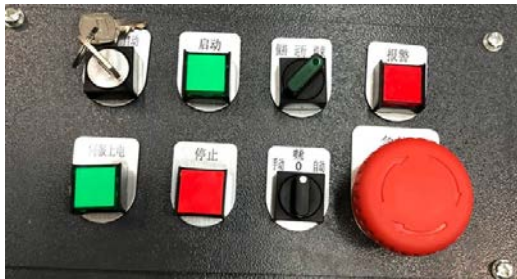
Figure 73:Control Panel 控制面板
