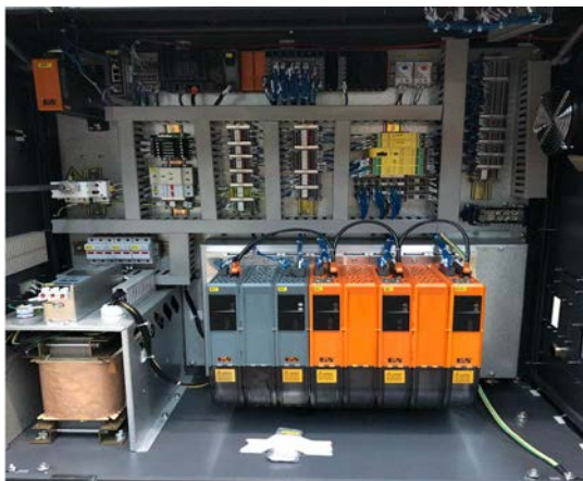
Figure 68:Cabinet interior 电柜内部
