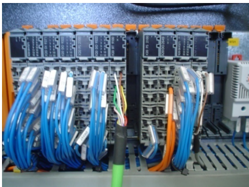
Figure 35: SINCONV connection SINCONV 的连接
